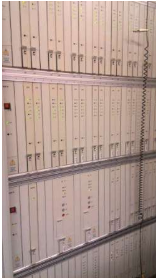
Gambar 3.4 Shelves&Racks ZTE ZXJ10
